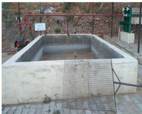
Figure 5 Image showing west water treatment Plant
